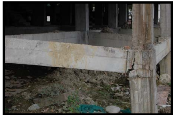
Examples of buildings under construction at the time of the earthquake (Dujiangyan, Sichuan Province, China).
